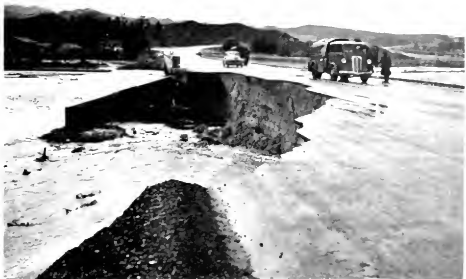
One lane of approach to bridge over Santa Clara River on U. S. 6 damaged
